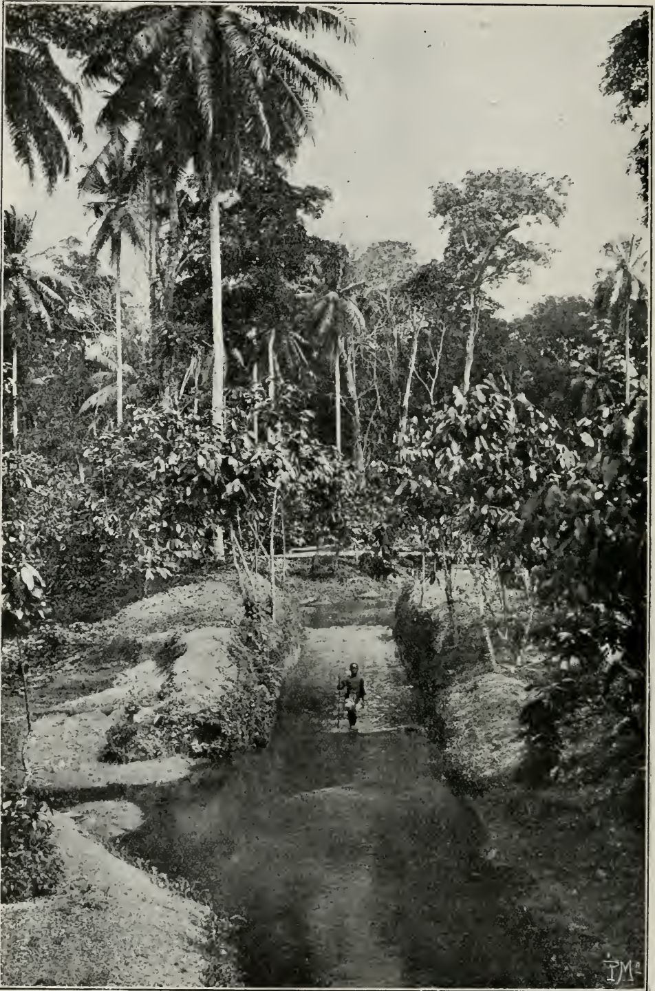
FIG. 32.—CUTTING MADE IN BED OF RIBEIRA DUMÚ, ROÇA SUNDY, FOR THE FREER FLOW OF ITS WATERS.
